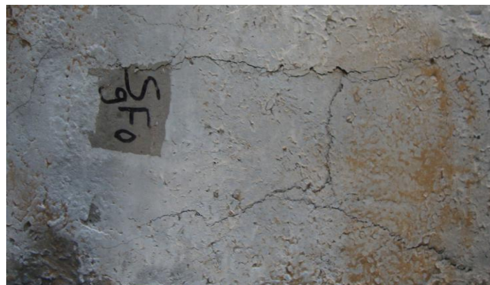
Plate 2. Top failure surface of SCC slab without fibres.
