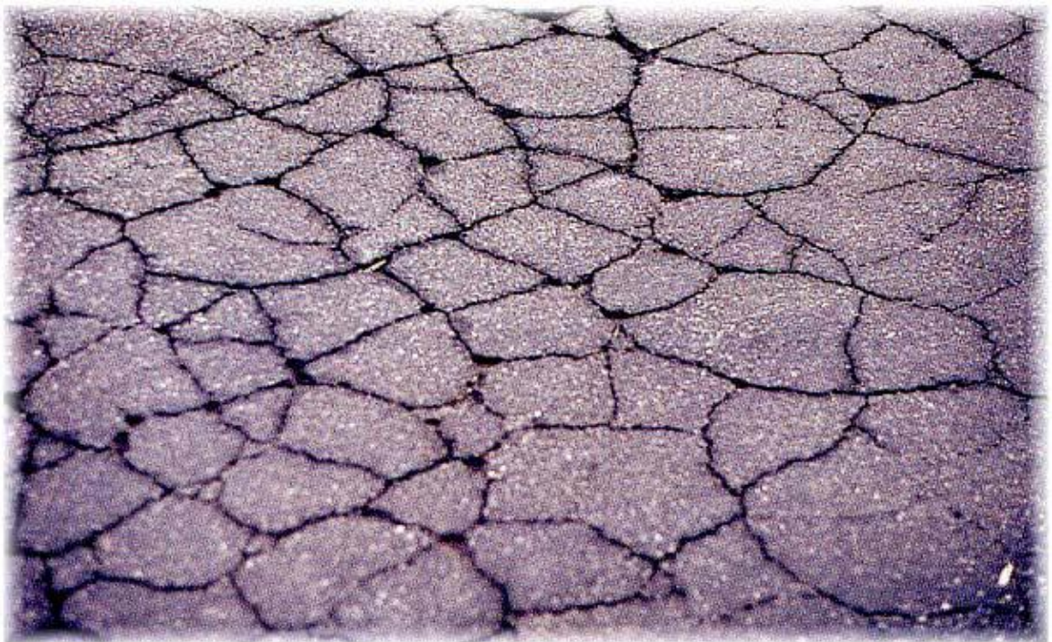
Figure (12) Flexible pavement distresses fatigue cracking (Bahia)
