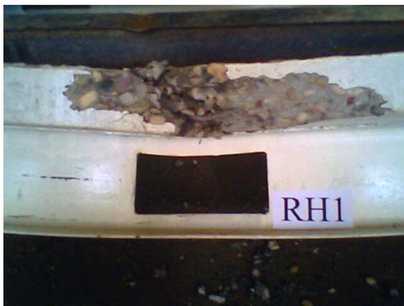
Figure (5): Opening RH1 of Beam CB1 at Failure
