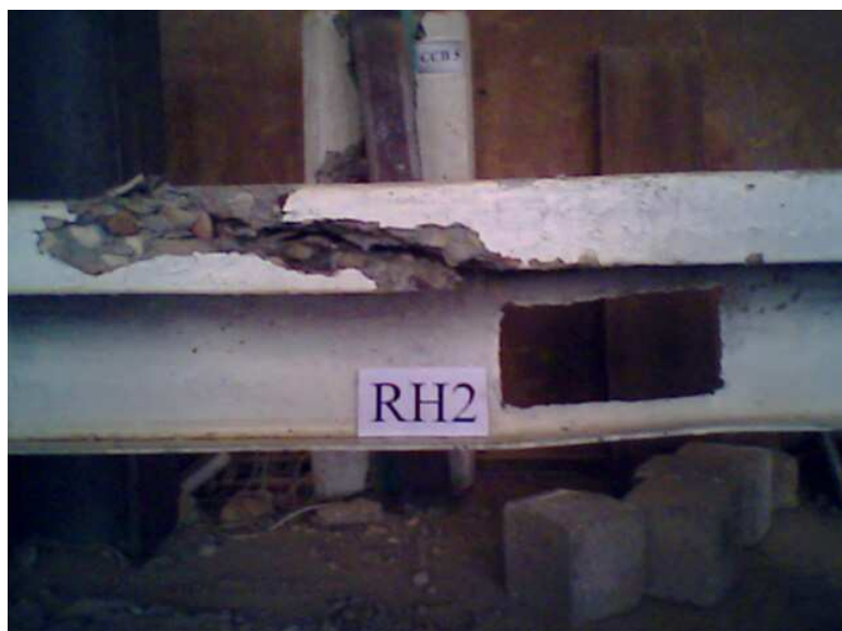
Figure (7): Diagonal Cracking at Hole RH2 of Beam CB2
