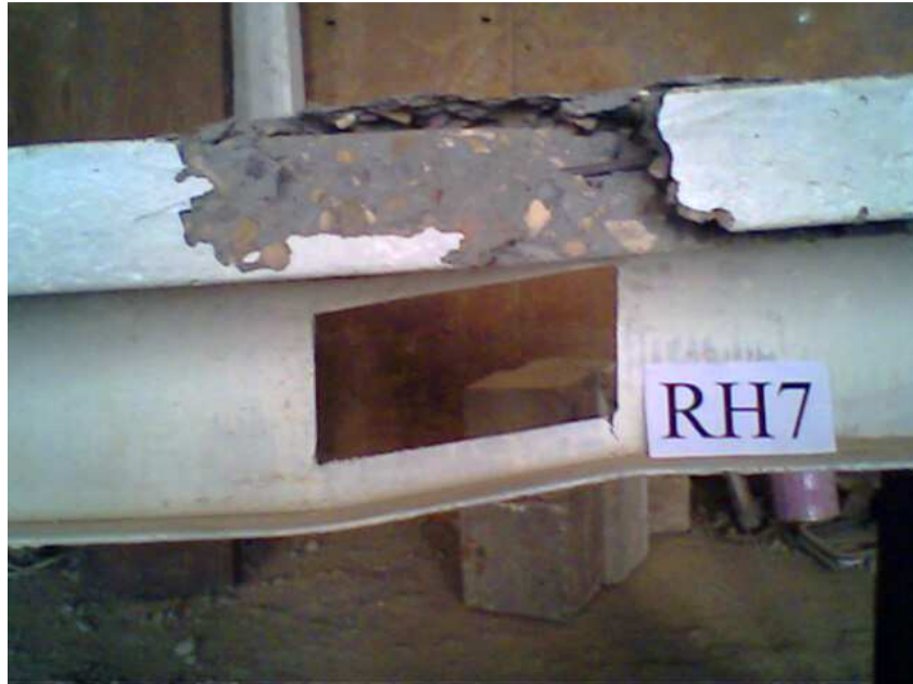
Figure (10): Failure at Opening RH7 of Beam CB4
