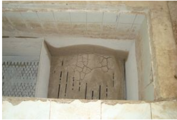
Figure 13. The phenomenon observe where about 30-cm thick scum is accumulated at tank
