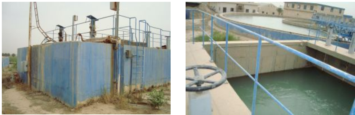
Figure 6. Coagulation and Sedimentation
