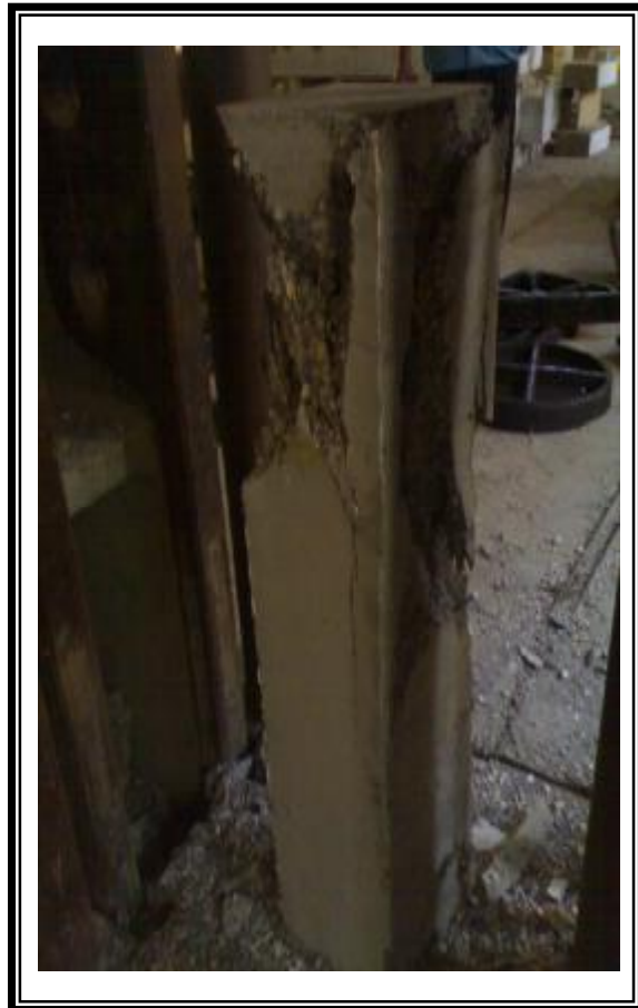
Figure (10) Failure Mode of Column A 3 B 1 C 2
