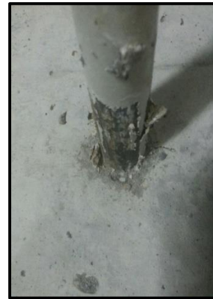
Fig. 10 - Slip of dowel bar for coated lubricated dowel bars at concrete contains 0% CR
