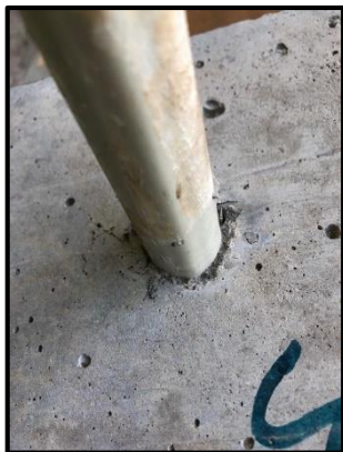
Fig. 9 - Slip of dowel bar for coated lubricated dowel bars at concrete contains 6% CR
