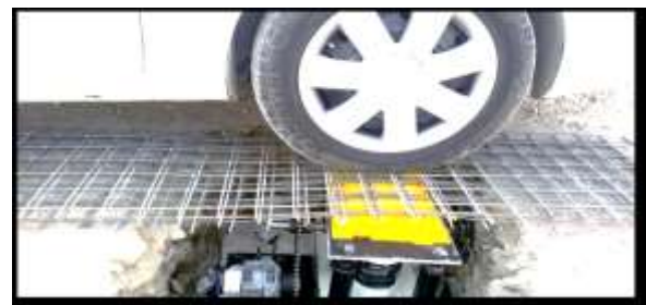
Figure 11: Passage of front wheel over the speed breaker mechanism
