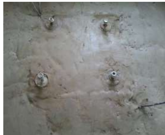
Plate 5: Preparation of a clay surface prior to connecting the pile cap to piles
