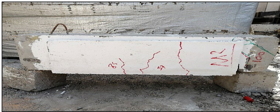
Figure 9: Cracks in reinforced concrete beam strengthened with type 2 Ferro-cement layer
