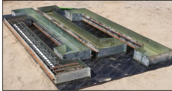
Figure 3: Reinforcement cage with a PVC pipe inside the formwork of each group
