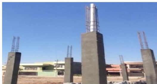
Figure 1: Inner rain drainage pipe placed inside the columns Preparing the Column Specimens and Testing Program
