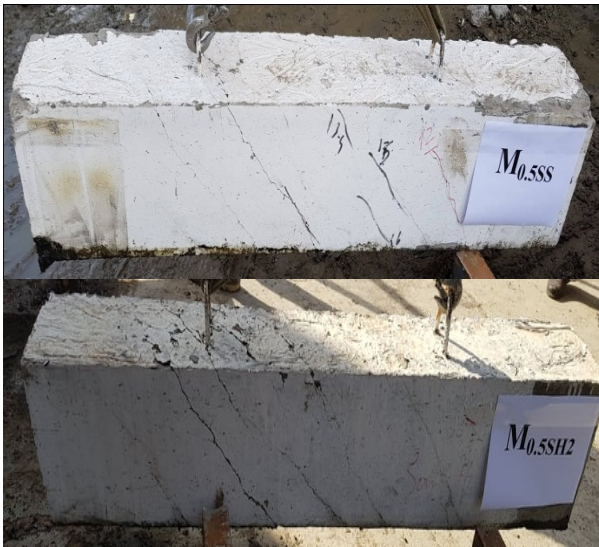
Figure 13: Crack pattern and failure mode for M_{0.5H} , M_{0.5S} beams
