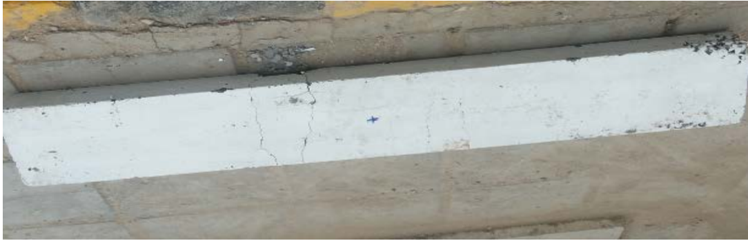
Figure (8.1) Cracks pattern after failure for slab SHC
