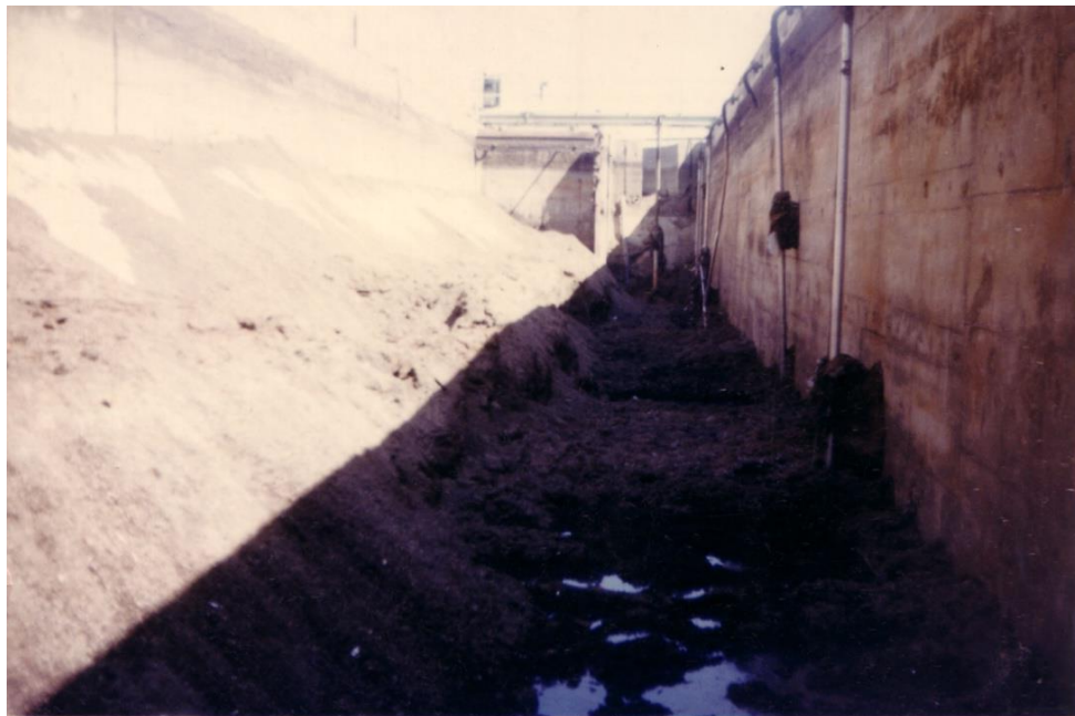
Plate (2) A dewatered AGC "location of Grit Mounds
