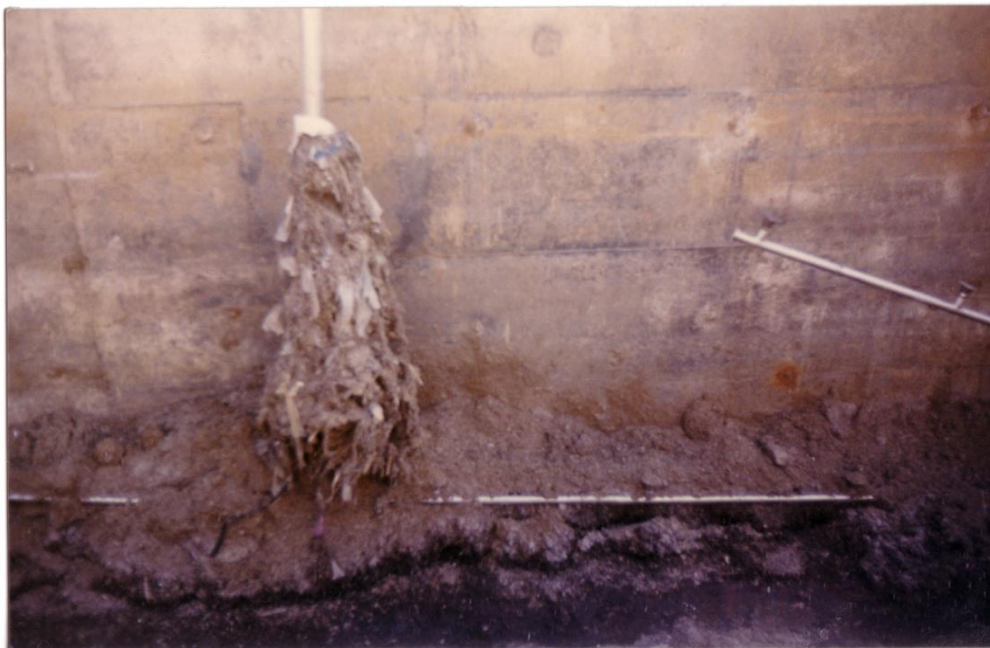
Plate (4) A dewatered AGC "Aeration Equipment's Clogging".
