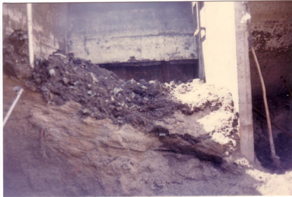
Plate (1) Accumulation of Grit Mounds at the Outlet Zone of a Dewatered AGC.
