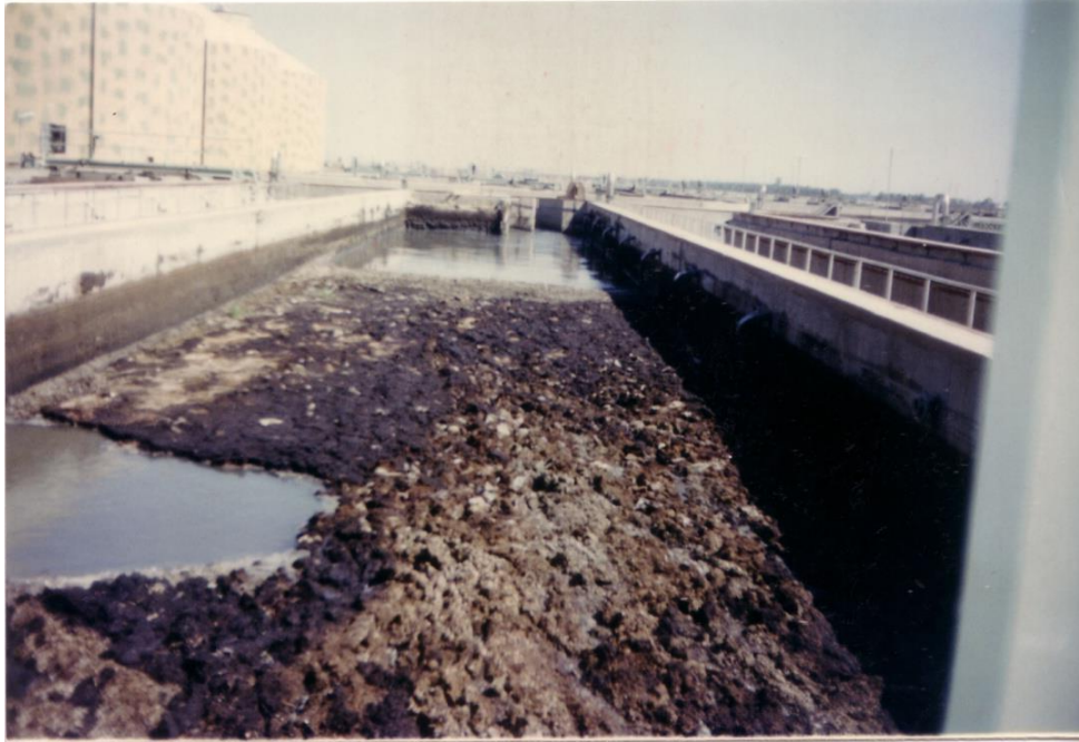
Plate (3) Scum Accumulation at the Outlet Zone of a Working AGC.
